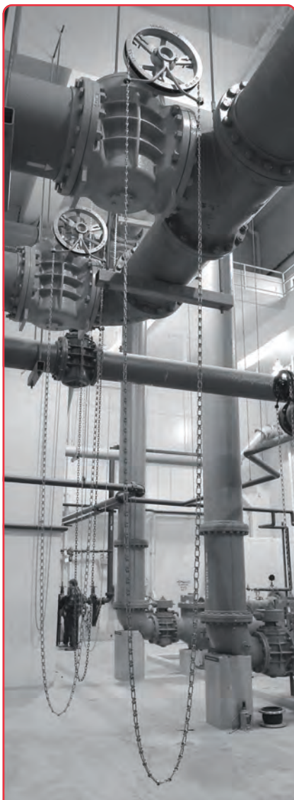
CHAIN FROM OVERHEAD CHAINWHEEL SHOWN IN PATHWAY.
