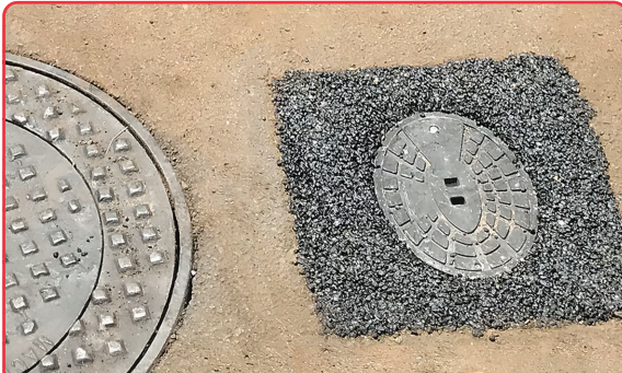
VAULT WITH REMOTE ANTENNA BOX.
